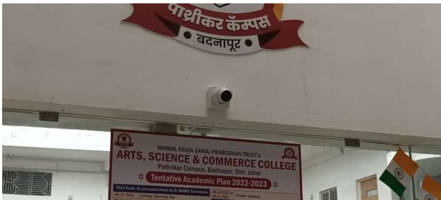
CCTV CAMERA AT ENTRY OF COLLEGE BUILDING
