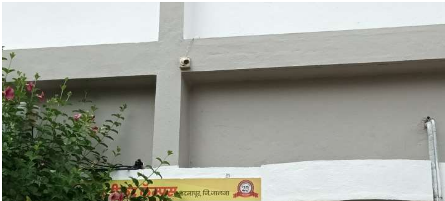
CCTV CAMERA ON COLLEGE BUILDING
